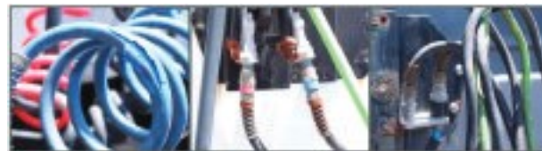
Damaged Jacketing, Rusted Springs
