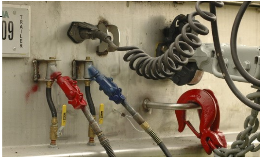
Trailer connectors that remain plugged into their sockets most of the time are not immune to corrosion. It may be even worse in there if you operate where corrosive deicing fluids are used.
