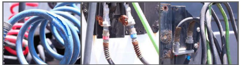
Damaged Jacketing, Rusted Springs
